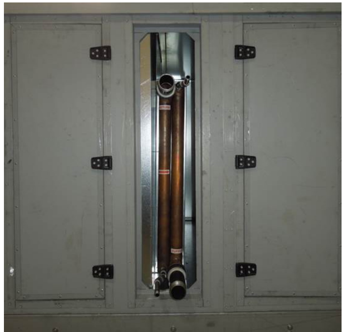
FIGURE 17: UNIT WITH CHILLED WATER COILS ▼
