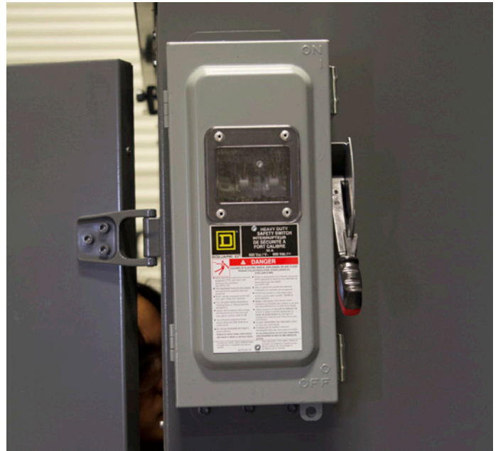
FIGURE 10: TYPICAL FACTORY SUPPLIED DISCONNECT ▾
